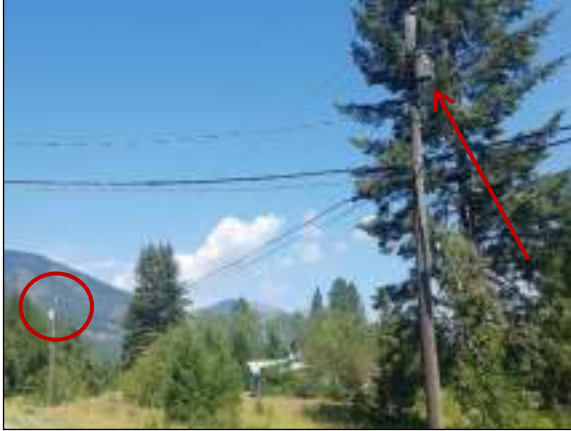
Photo 13. Power pole-mounted electrical transformers observed along West Creston Road.
